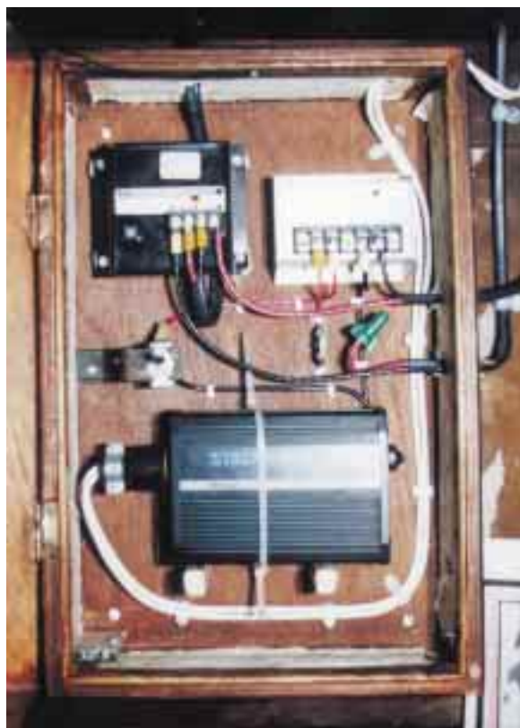
Below: A close-up of the power center on Lama Ngawang Zima's bedroom wall.
